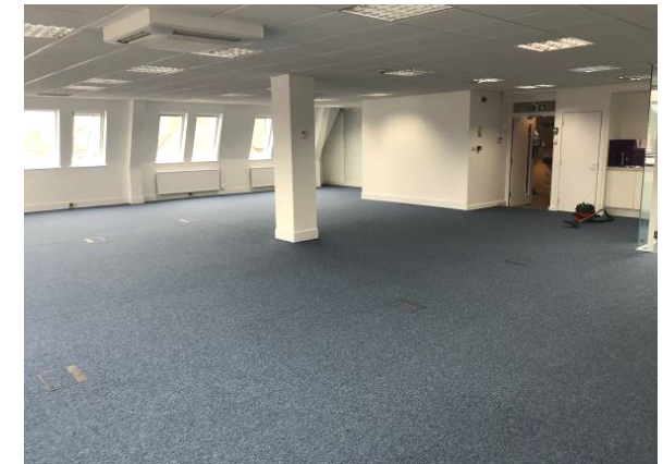
An example of another suite that was available on the 2 nd floor.
